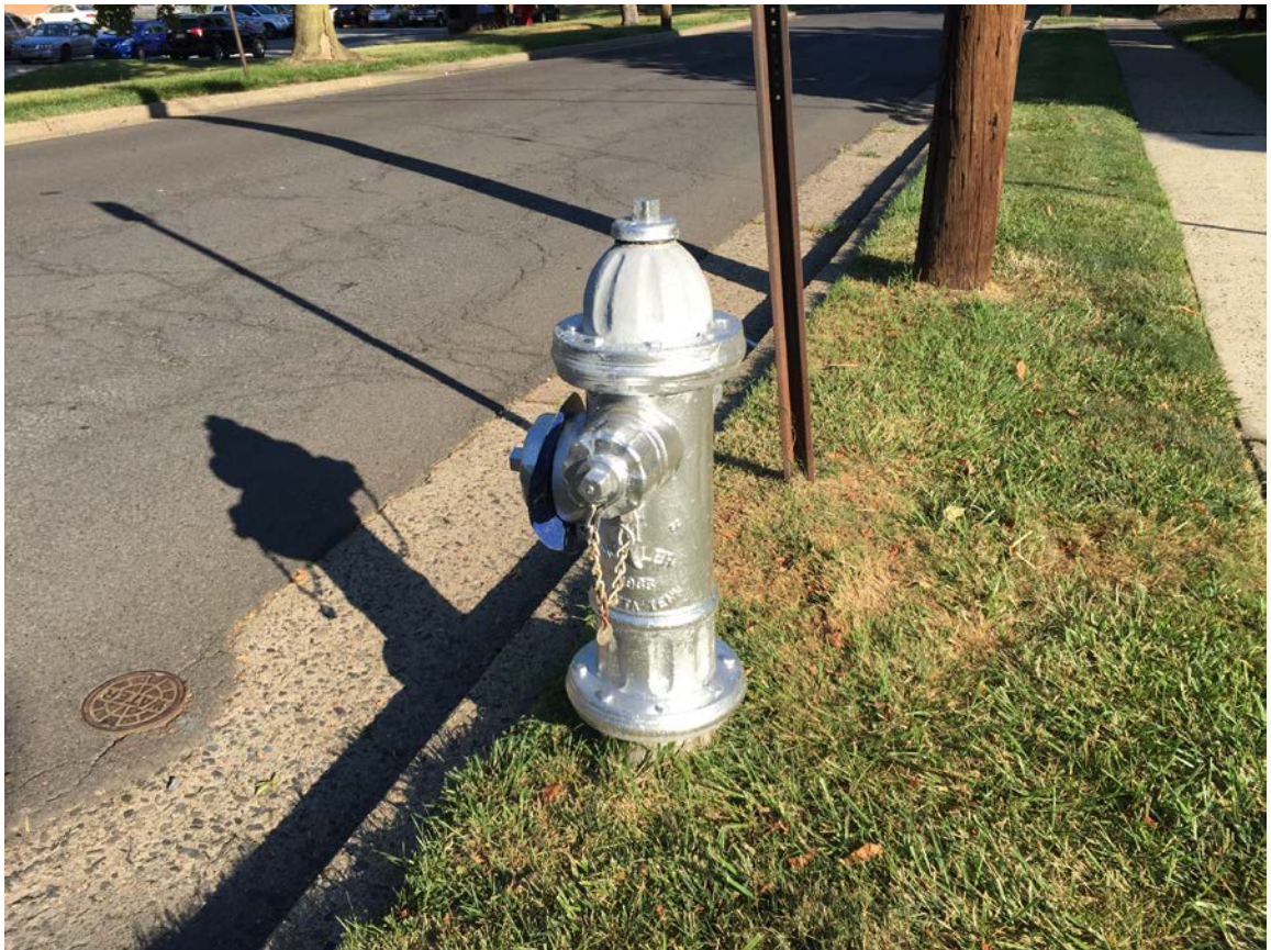
Above – A bolted flange hydrant for the breakaway stem. Typically the older style Mueller hydrants in the Township.
