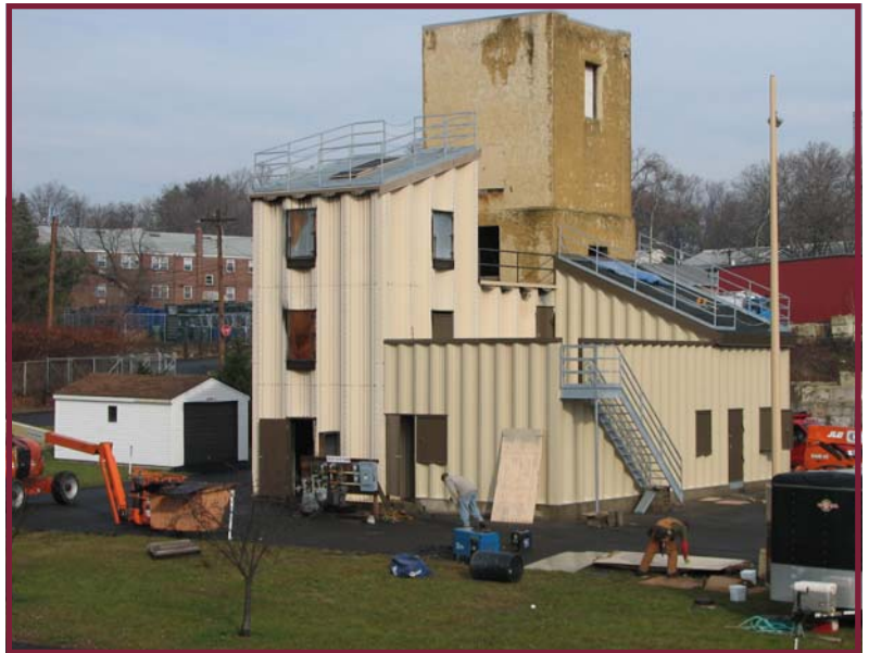
Construction continues on the new one-story addition to the ATFD's fire training facility.
